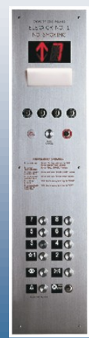
New ADA Compliant Car And Hall Fixtures
